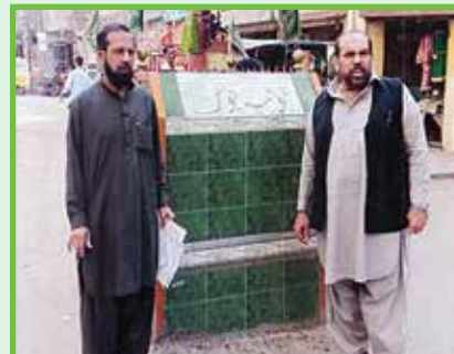
The Regional Director, Provincial Ombudsman Sindh, Karachi-South visited to verify the repair of road and laying of pipe line in Soldier Bazar No.02 Ghousia chowk, around Zainabia house, Roderick Street, Karachi.
